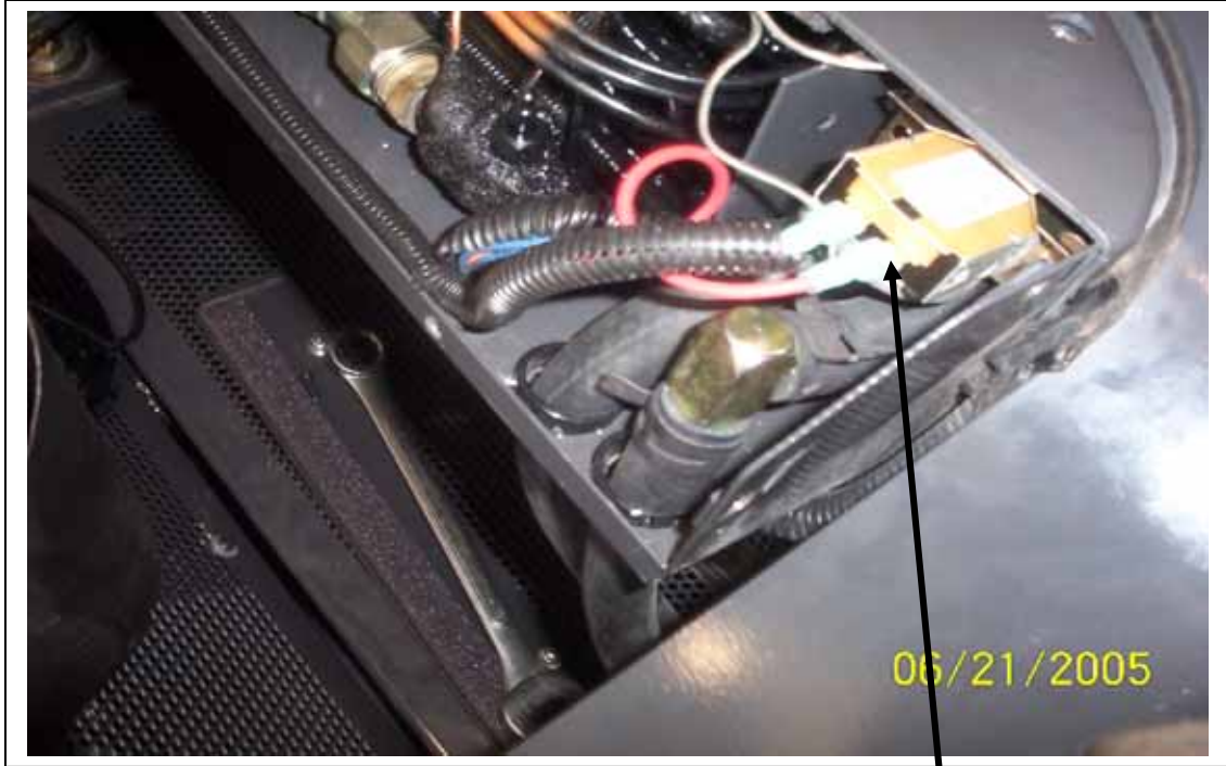
Thermostat located at the evaporator.
